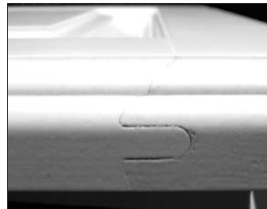
Example of end joint separation
